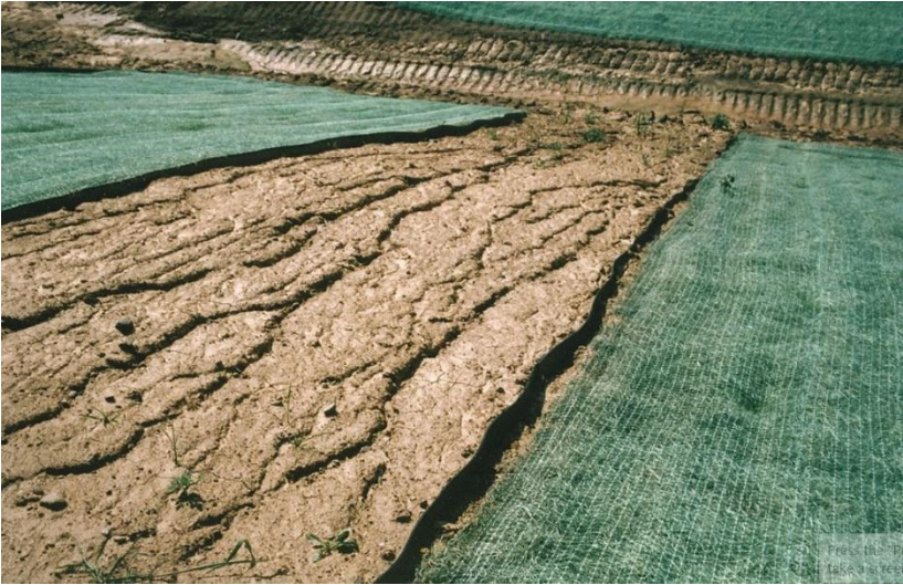
Figure #9. Coir Blanket Similarities with Fiber at Smiths Cove. 73
